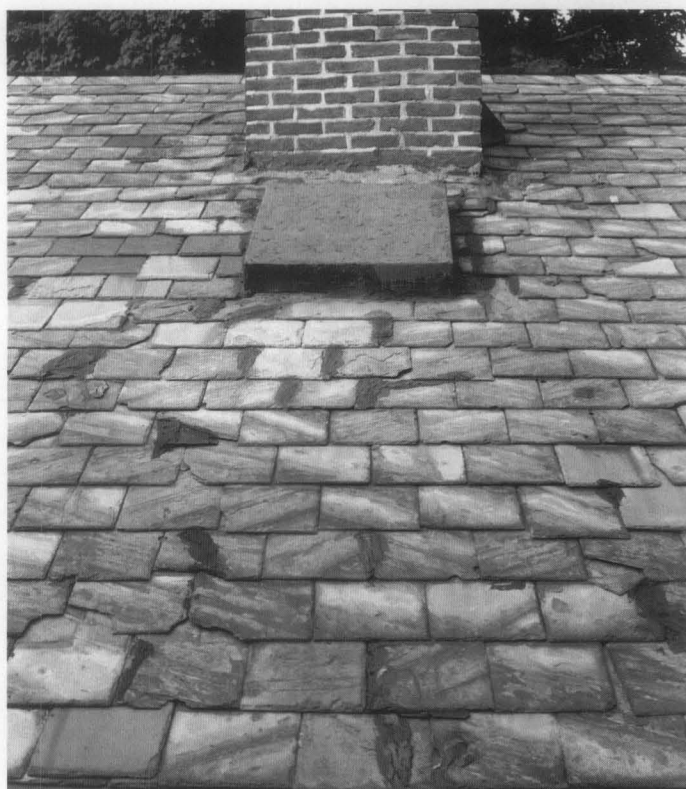
Figure 20. This roof has been poorly repaired numerous times in the past. The installation of mastic to seal out moisture has only exacerbated the problem. A timely repair and good maintenance could have extended the life of this roof.
