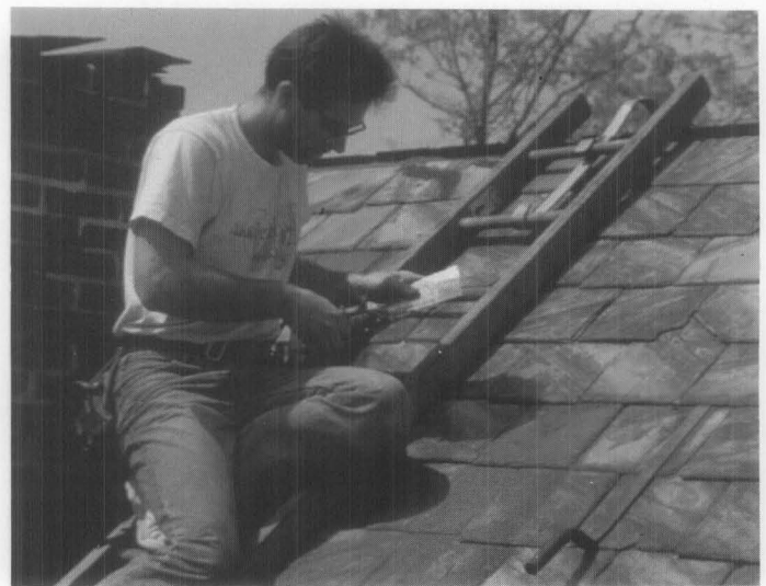
(d) A copper bib is formed to protect the newly created nail hole.
