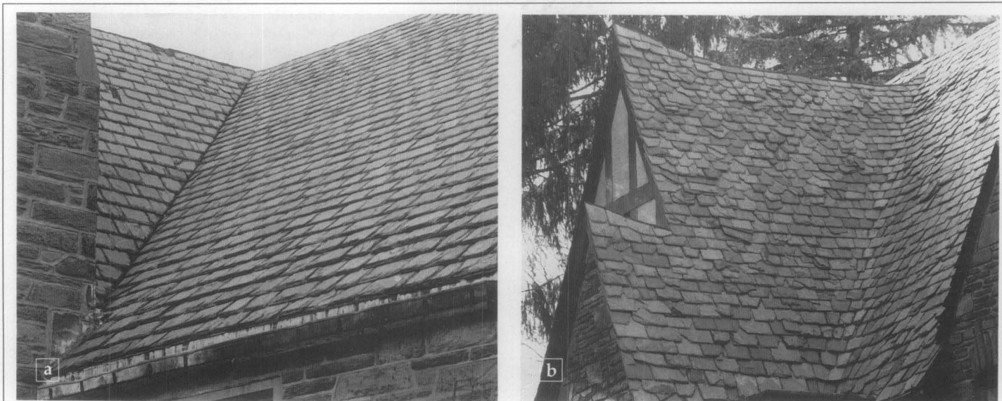
Figure 9. Valleys are formed at the internal angle of two roofing slopes. Flashing is often placed under the slate to increase moisture protect at this vulnerable joint. Shown in (a) is a closed valley where the slates are held tight to the valley line. (b) illustrates of a round valley where the transition between the two slopes is a continuous curve. It requires careful workmanship and an experienced roofer.
