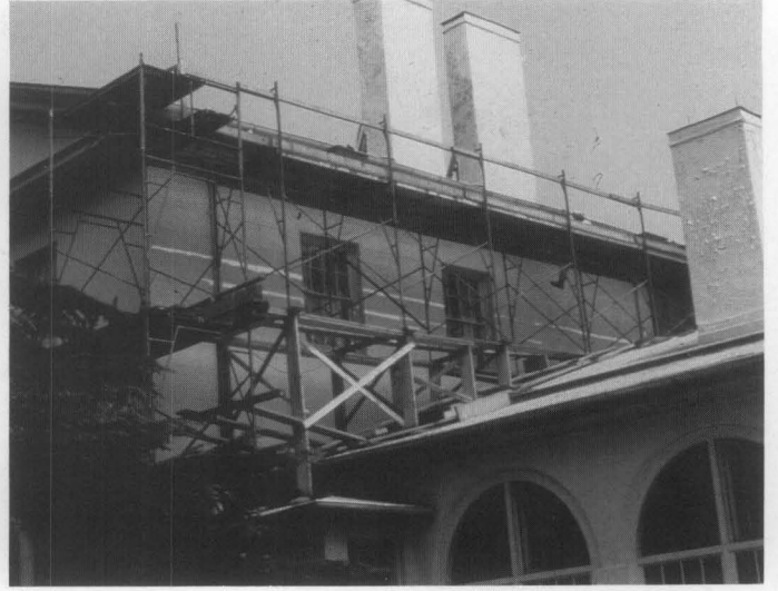
(b) Scaffolding was installed early to document existing conditions to determine extent of work.
