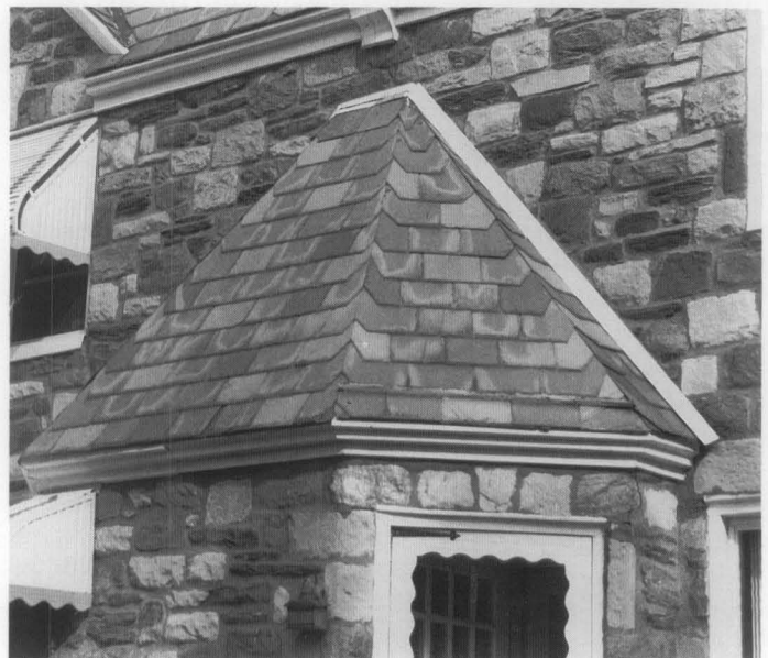
Figure 14. The white blotches on these Pennsylvania Soft-Vein slates indicate areas where gypsum is leaching out onto the surface of the slates.
