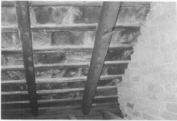
Figure 15. View of the underside of slates laid on open sheathing shows that delamination and flaking is just as bad or worse on the underside of slates as on the exposed surface. This is why most slates cannot be flipped over for reuse.
